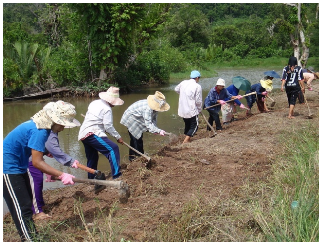
Figure 6: Villagers regrading shrimp pond embankment to increase the area where mangroves will grow. Before this work, the pond had steep walls and a flat, poorly drained bottom. This work produced more area at an elevation suitable for mangrove growth and improved the pond drainage.
